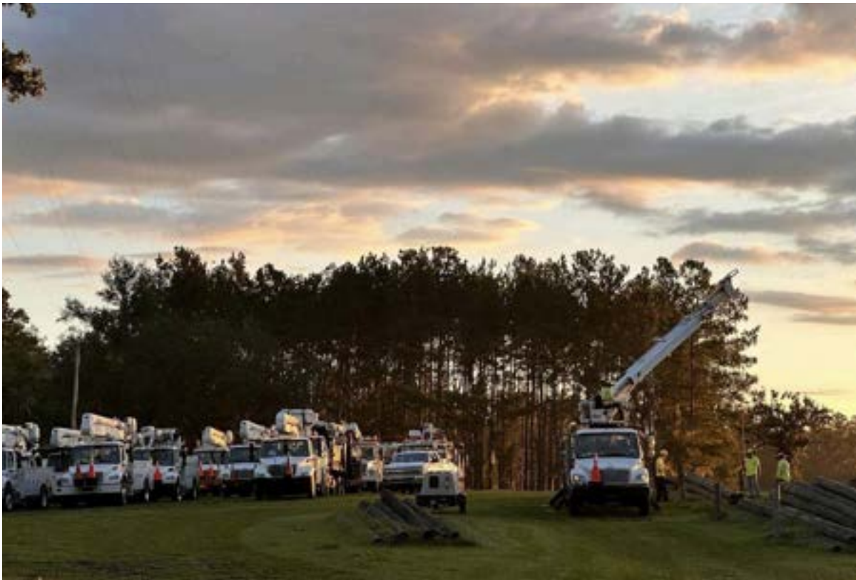
Photo: Tri-County Electric Cooperative
