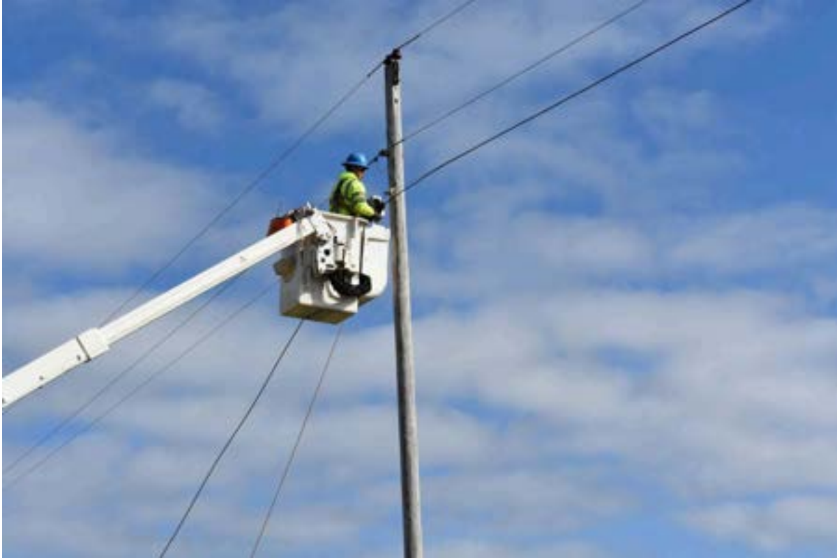
Photo: Osage Valley Electric Cooperative
