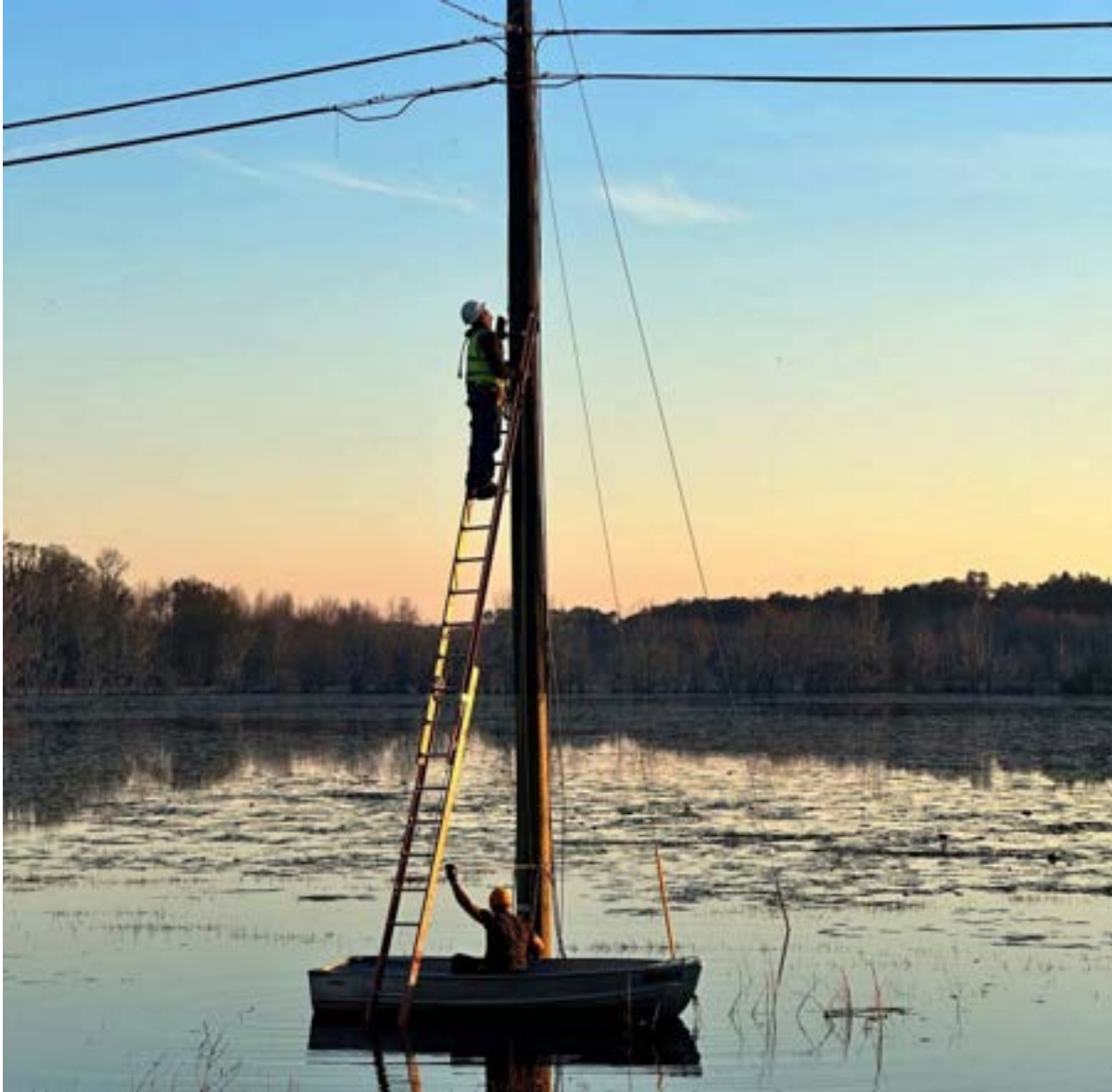
Photo: Tri-County Electric Cooperative
