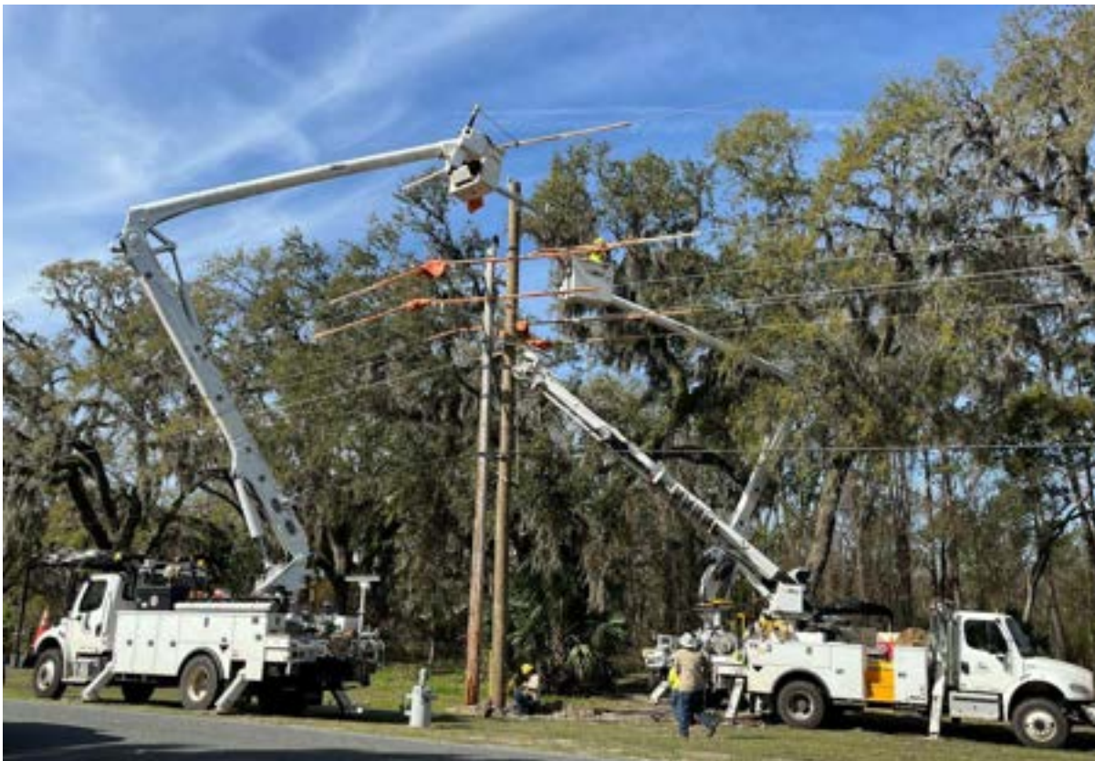
Photo: Tri-County Electric Cooperative
